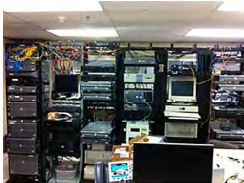
A typical small server room; this one at Stanford University
