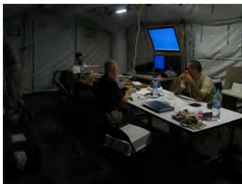
Test of advanced lighting controls in a military shelter at Crimson Viper technology demonstration.
