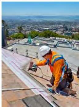
A worker installs a cool roof on Berkeley Lab's Advanced Light Source.
