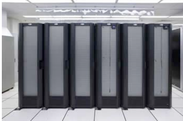
Passive rear door heat exchanger devices help optimize energy efficiency in a data center at Lawrence Berkeley National Laboratory.
