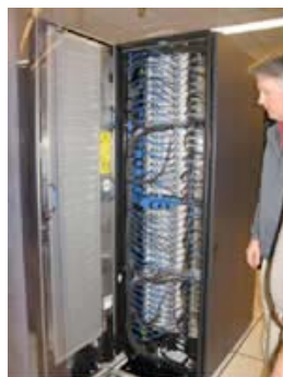
The opened back of a server rack with rear door heat exchanger devices installed.
