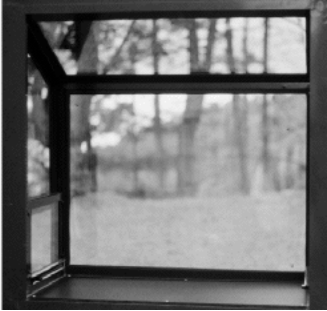
Figure 1: Greenhouse windows, such as this one, and other projecting fenestration products can now be modeled more accurately with THERM 2.0.
